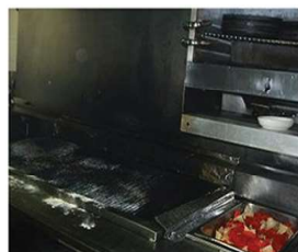
After fire suppression
